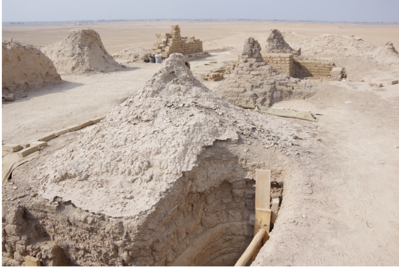
Phases of implementation: soil consolidation (left) | cleaning of the eroded layers (centre) | emergency-securing addition to the masonry with earth blocks and earthen masonry mortar according to the characteristics of the original (back). © J. A. Blaschek (ZRSI)
