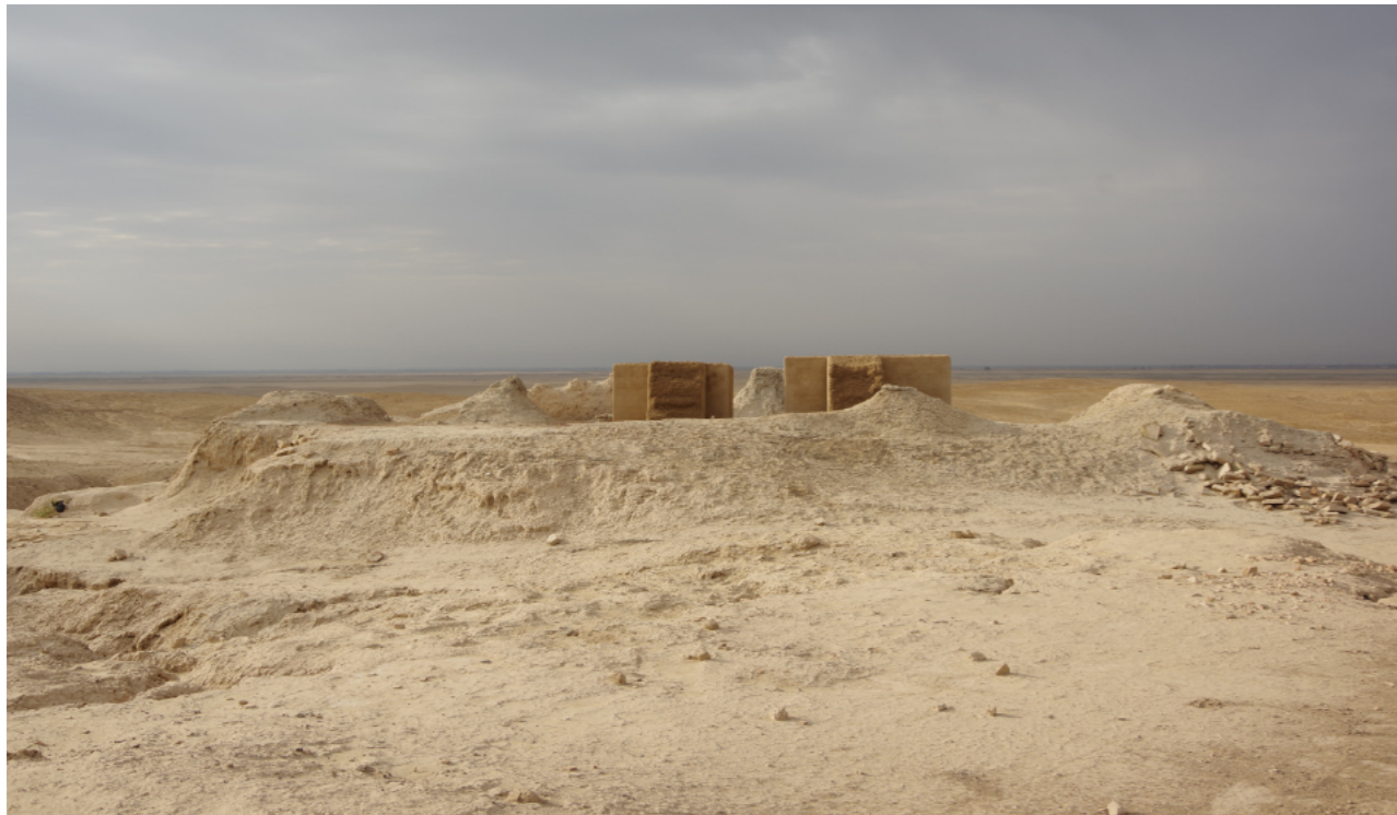
Completion of the supplementary works in autumn 2022, view from NE © J. A. Blaschek (ZRSI)
