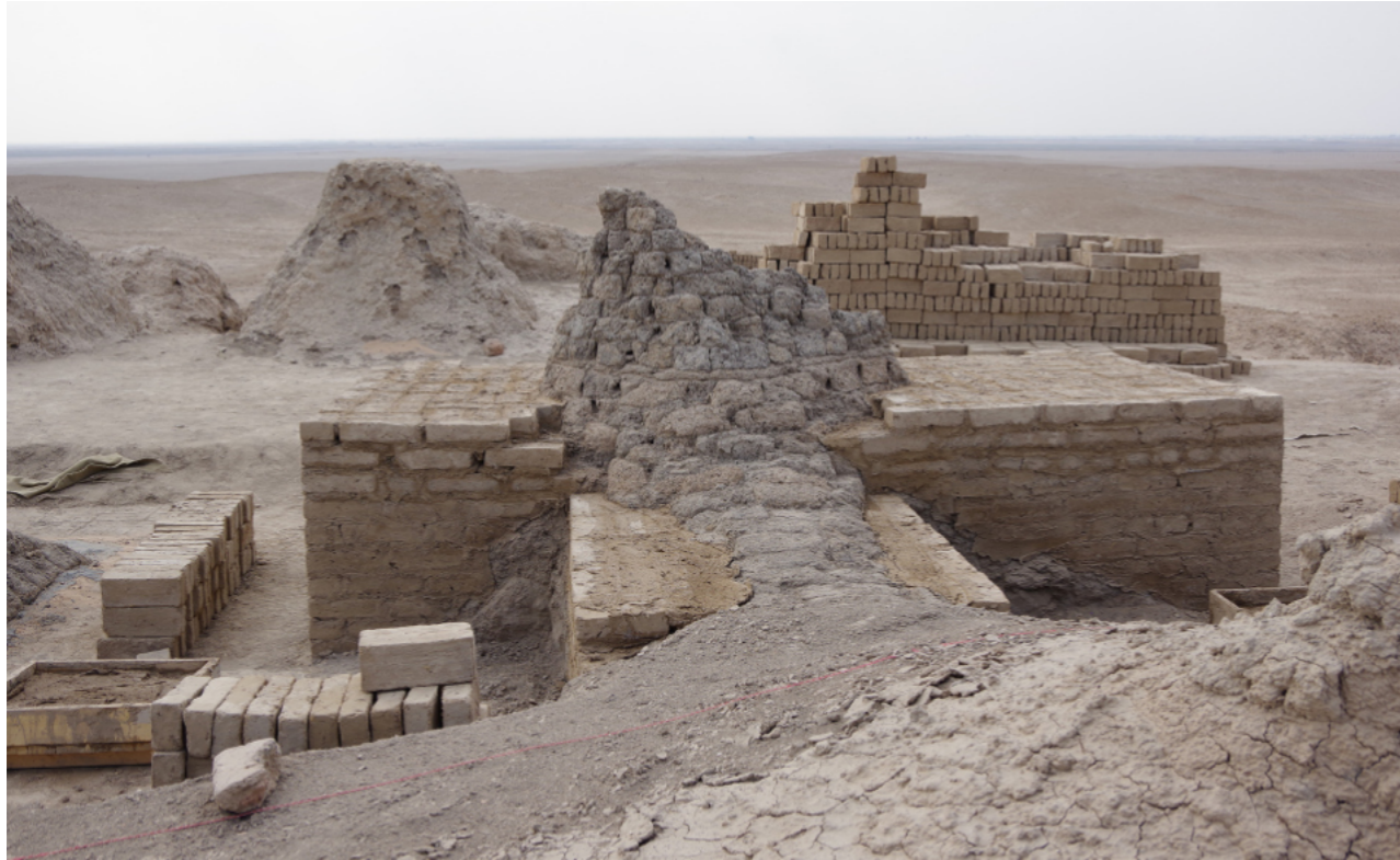
Titel: 3 phases of emergency conservation | interlocking sheathing of the original finding according to detected remains at the masonry base (front) | exposure of the solid core (centre) | ground consolidation (back). Adapting to the remains of original masonry made of earth blocks © J. A. Blaschek (ZRSI)
